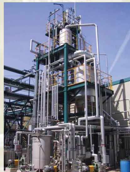
Dioxane Removal System
