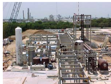
Huish MES plant in Houston, photo courtesy Chemithon
